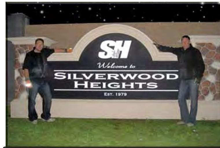
Sign technicians from Magnetsigns North work late into the evening to install the Silverwood Height New Community Boundary Sign
